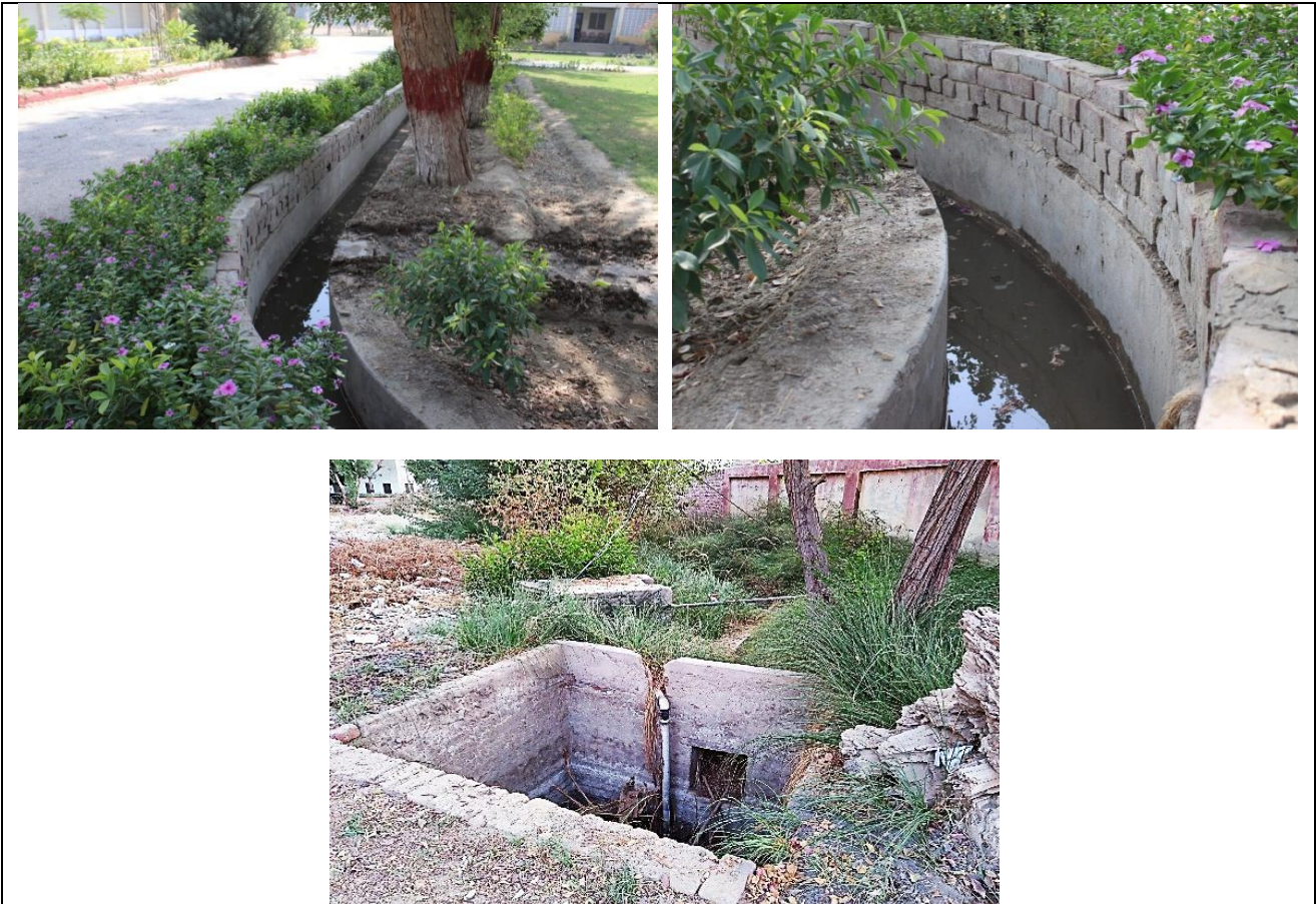
Snapshots of Sewerage Disposal at The Benazir Bhutto Shaheed University of Technology & Skill Development Khairpur
